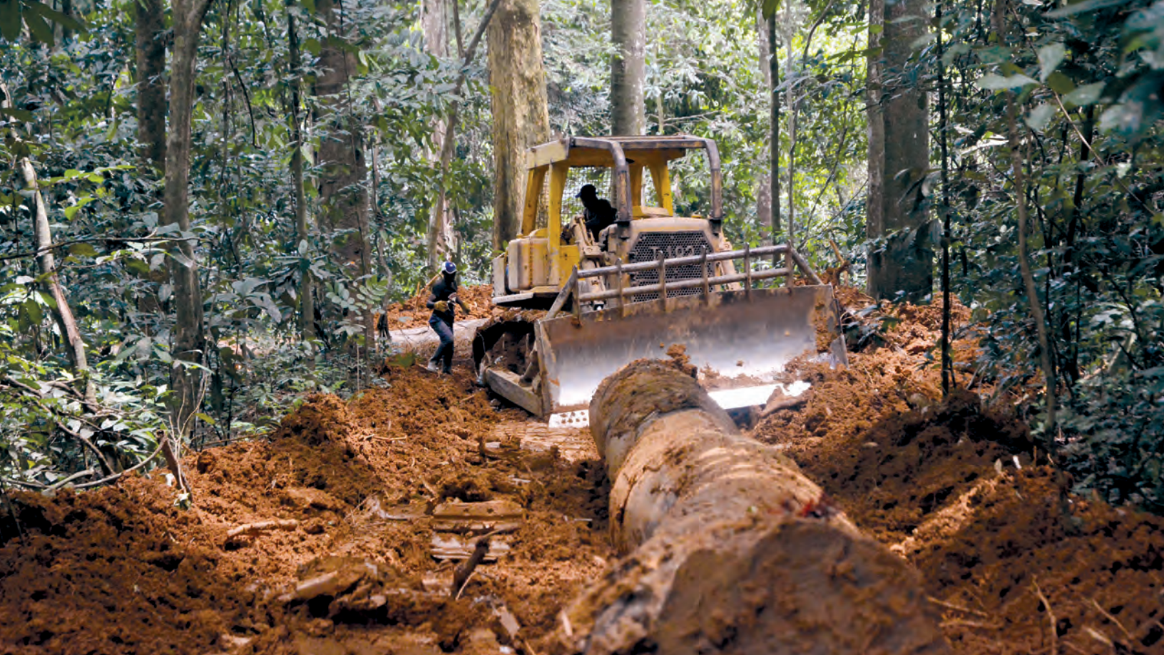
A bulldozer opening a secondary logging road in a forest concession in Gabon. Source: ANPN
