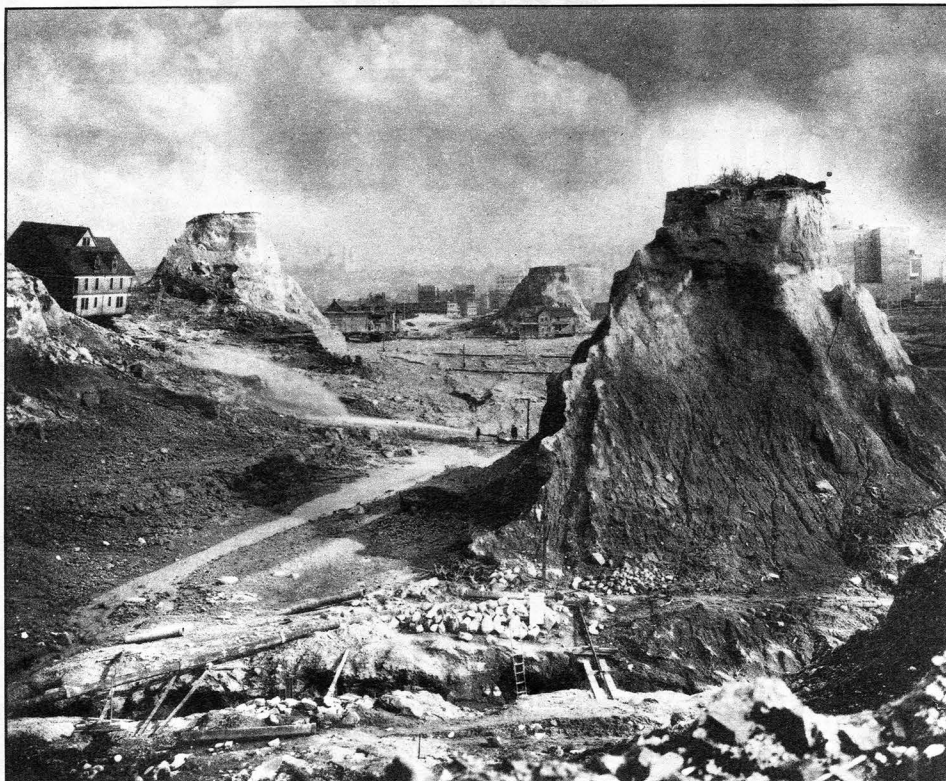
Water hoses helped carve this 1910 scene of the Denny Regrade. The view is south from Bell Street.
